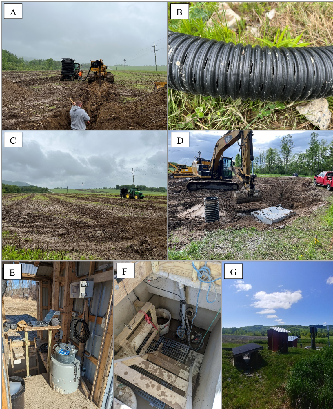
Figure 1. (A) Installation of systematic tile drainage into East field in June 2023; (B) section of drain line PVC with small perforations for drainage water to flow into (C) field immediately following installation of tile laterals, prior to any tillage or other soil disturbance (D) installation of concrete tank at the field edge where tile outlet empties into for monitoring; (E) equipment structure located above concrete tank with tile main outlet; (F) looking down stairs into concrete tank; (G) surface drainage flume (foreground), surface drainage equipment structure (middle ground), partially obscured tile drainage equipment structure (background); Quantifying Long-Term Agronomic and Water Quality Impacts of Tile Drainage in Northern New York; NNYADP
