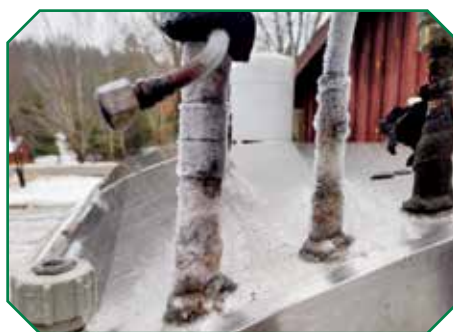
Right: Smaller DIY chiller connected to cooling plate submerged into open top sap collection tank.
