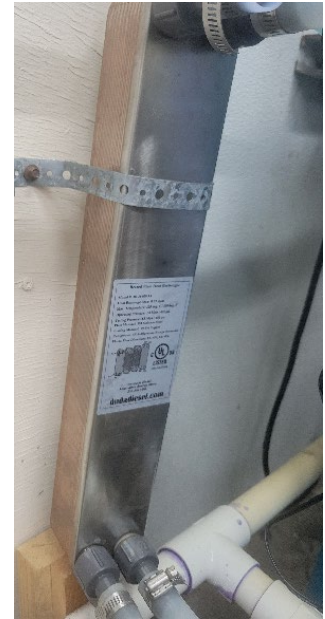
Figure 6. Plate Heat Exchanger connected to RO and glycol chiller
