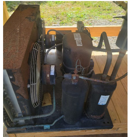
Figure 3. Compressor unit with condenser used for chilling and pumping refrigerant into the chilling tank in Figure 2
